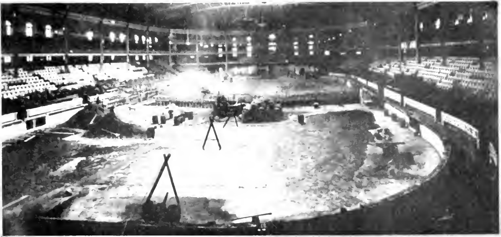
FIG. 29. ON JUNE 11 THE MECHANICAL WORK ON THE POOL WAS BEING DONE. THE WATER MAINS WERE BEING LAYED IN PLACE.
